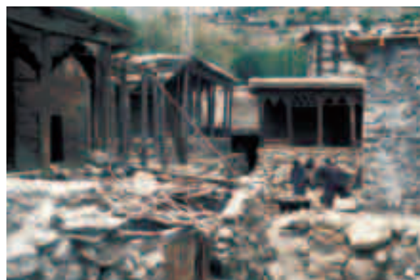
The “jataq” in Ganish before and after completion of the restoration works. In the background, one of the restored old watchtowers.
