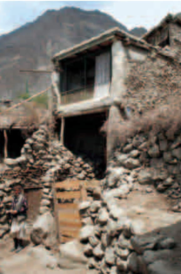
Partially collapsed traditional housing structures were typical of early conditions found in Karimabad.
