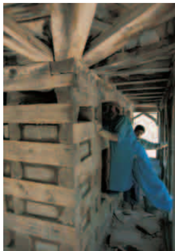
Below: Local craftsmen work on the re-assembled and restored “astana” of Sayyid Mohammad in Khaplu, one of the first “demonstration projects”.
