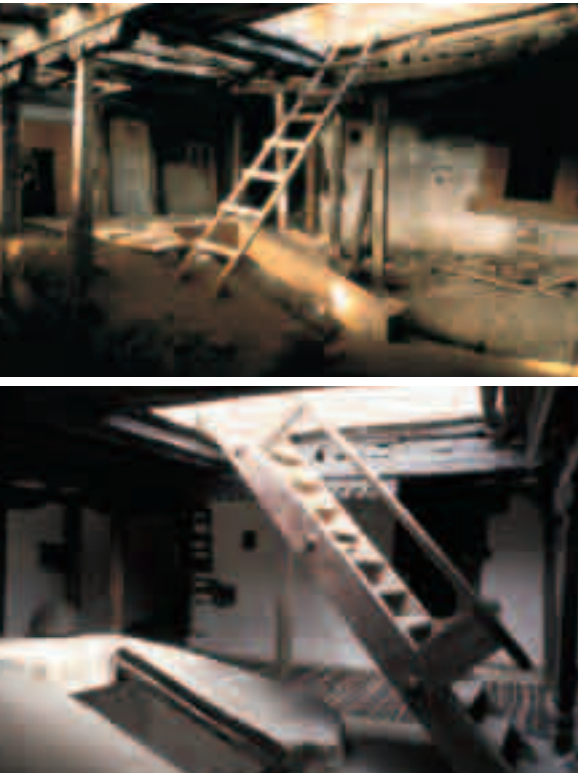
The central first floor arrival lobby of the Baltit Fort before and after restoration. The stairs lead up to the second floor terrace and the royal dais.
