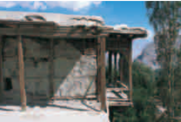
Rear facade (below) of the 19th-century Khaplu Palace and side balcony (above), all in existing condition. This building is another candidate for restoration.
