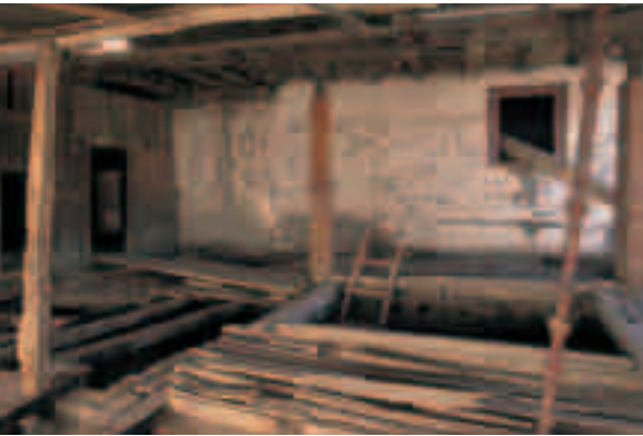
Stripping the interior of the building “to the bones” in order to analyse structural defects.
