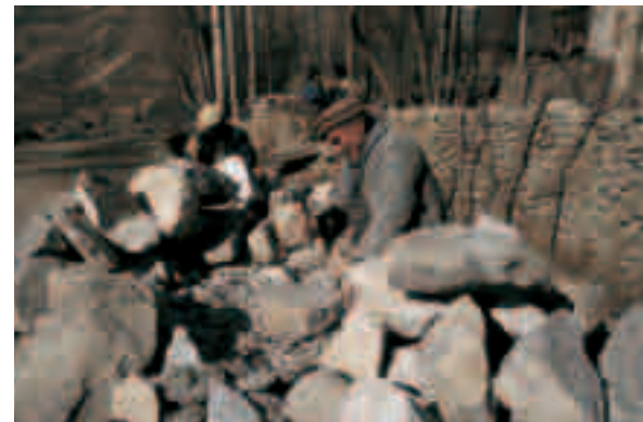
Community participation: Digging channels into the steep, rocky slopes of Karimabad for the underground sanitation system and preparing stones for house rehabilitation projects.
