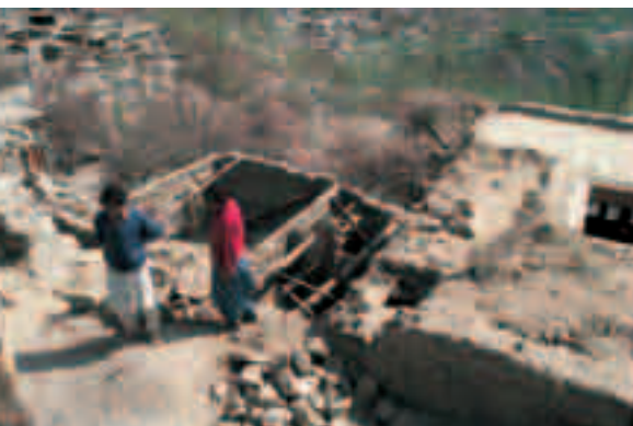
The terraced village of Baltit/ Karimabad from above, with house repair in the foreground.
